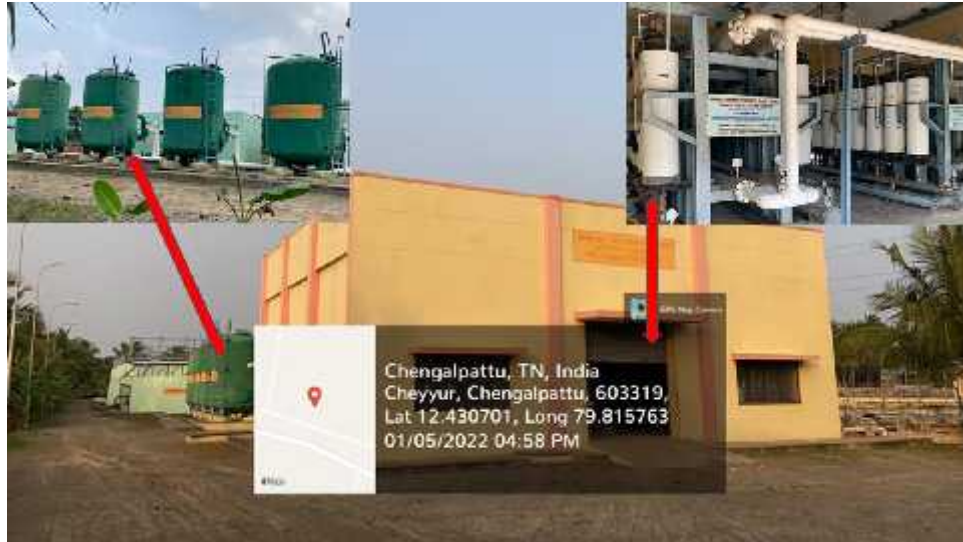
Sewage plants and multi grade filters in the campus
